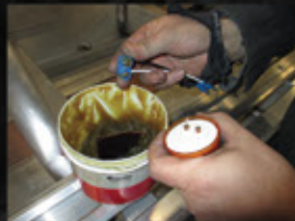
Extra Di-Electric Grease Added
